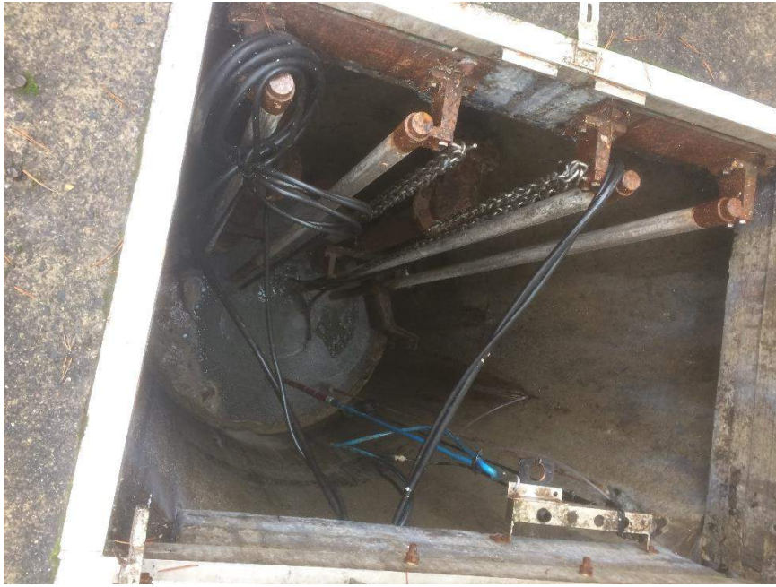
Influent Lift Station
