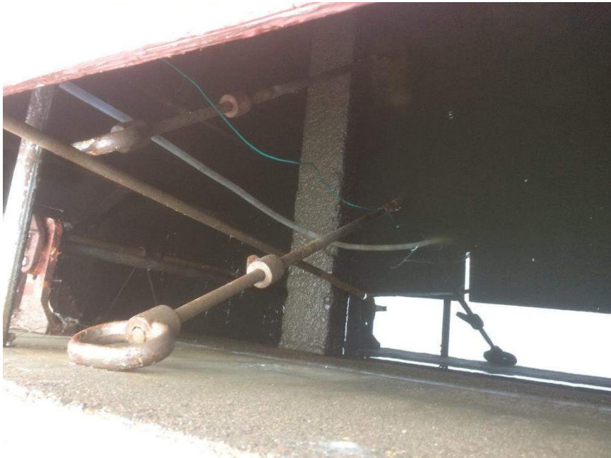
Splitter Box Upper Chamber
