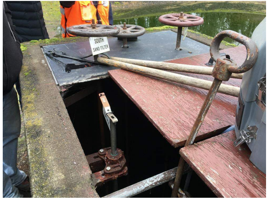
Splitter Control Valves
