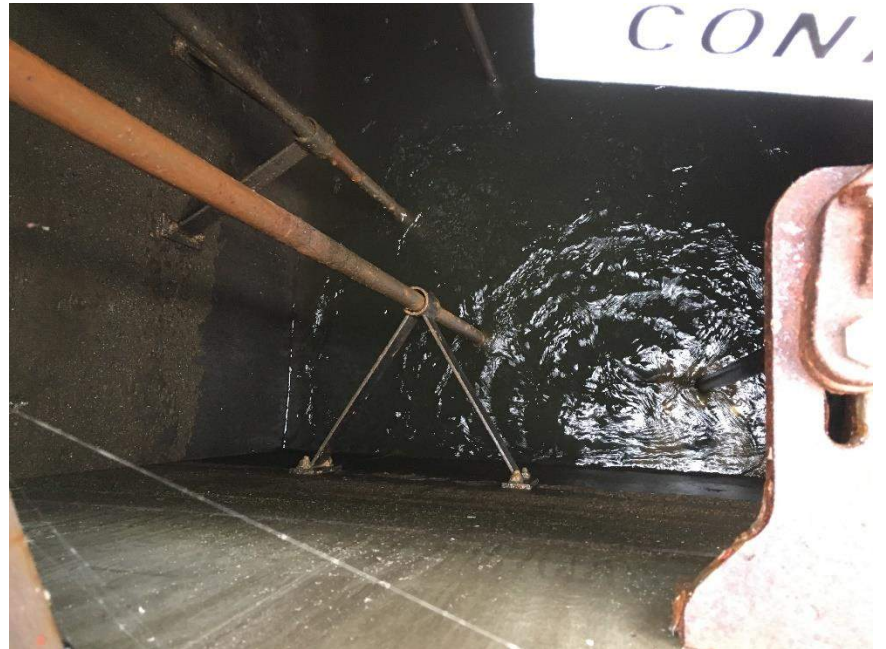
Splitter Box Lower Chamber
