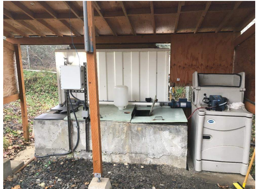
Radio, Flow Meter, and Autosampler
