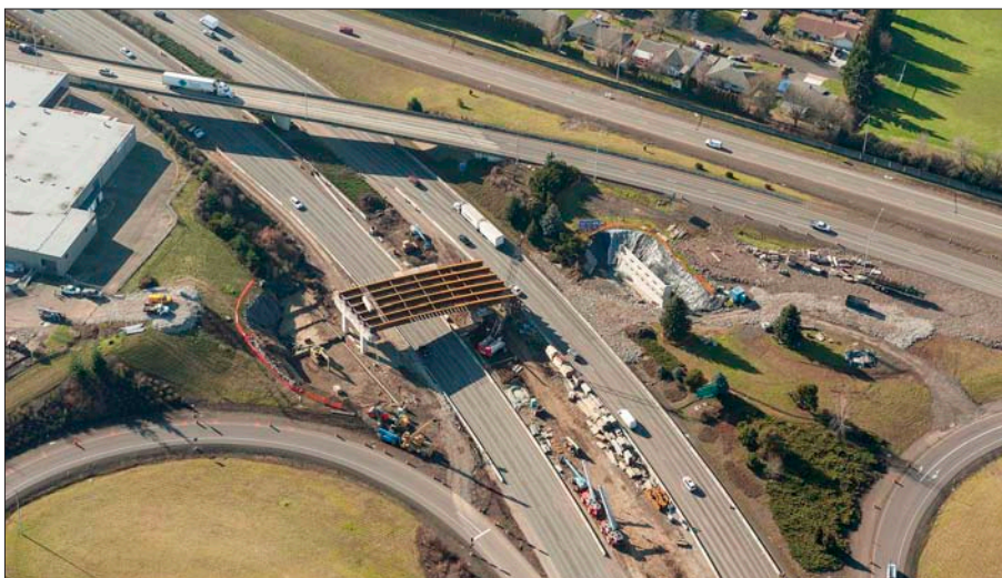
This photo, taken Jan. 21, 2014, shows the new girders placed over the northbound lanes of I-205. The girders are the support beams for a new overpass which will connect SE 82nd Drive with SE 82nd Avenue. Photos courtesy of ODOT
