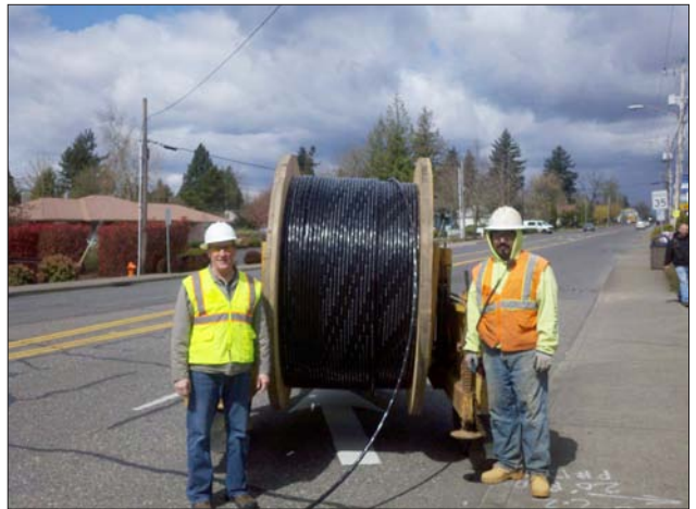
Workers install fiber as part of the Clackamas Broadband Express. The project was finished in October 2013.
