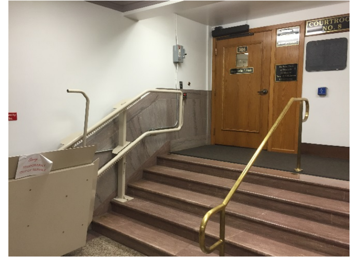
Stairs up to courtroom and non-functioning lift due to inadequate existing wall bearing capacity
